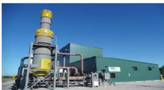
Landfill Gas recovery plant
