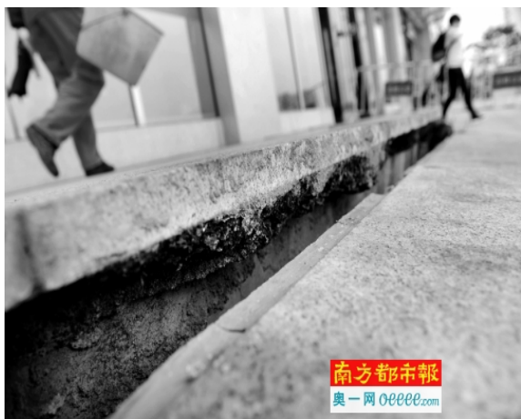
2016.01 Guangzhou Differential settlement
