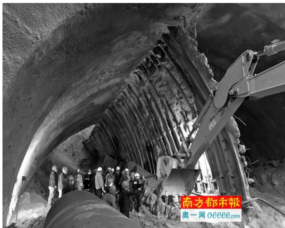
2017.02 Jiangmen Tunnel collapse 1 dead
