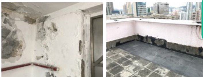
Typical examples of disrepair in Hong Kong's older residential buildings
